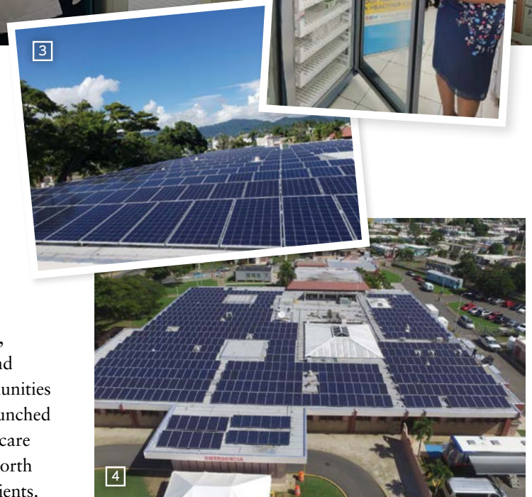
3 4 The Direct Relief-funded battery and solar power system at Family Health Center in Arroyo, Puerto Rico. (Courtesy photo)
